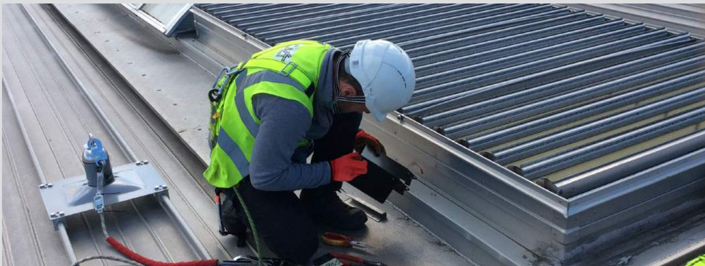
A UK service and maintenance technician maintains an actuator on a Colt ECO smoke control ventilator.
